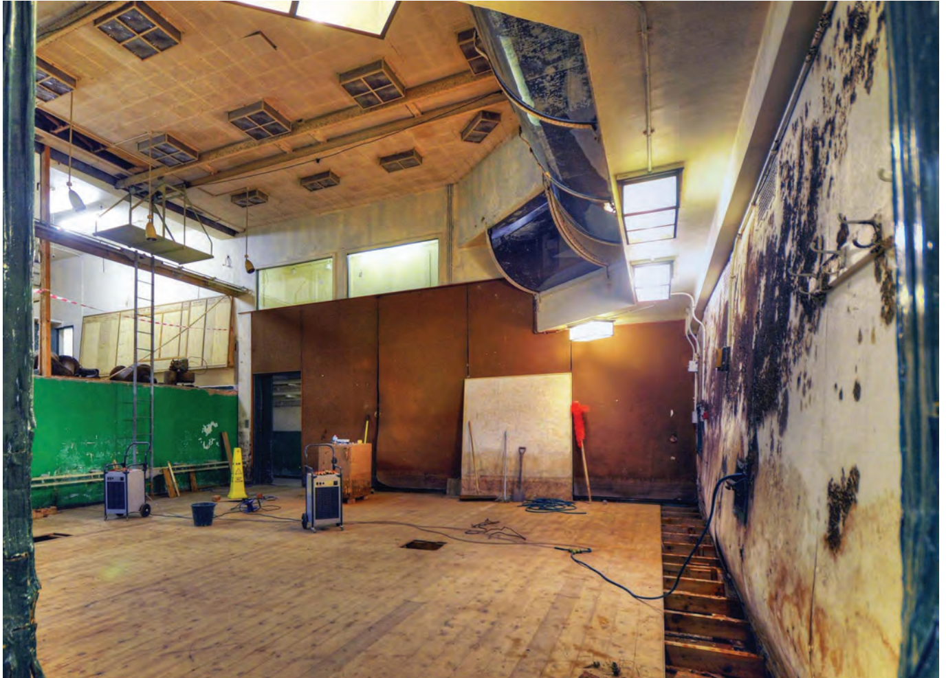
The new floor in the plotting room is nearing completion. Photo Colin Anderson
